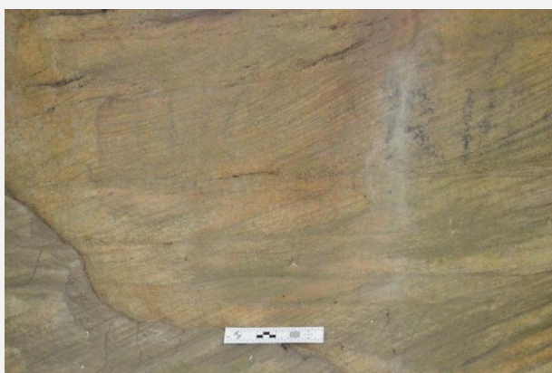
Plate 4: Overview photograph of graffiti on panel 3. See Drawing 1 for location at site (Source: Niche)
