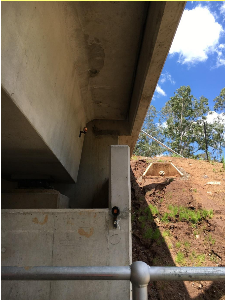
Fig. 2.12 Survey prisms located on abutment and bridge deck of Bridge Street Overbridge at 91.030 km
