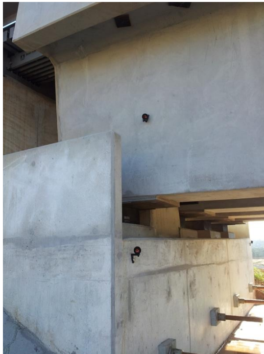
Fig. 2.8 Survey prisms located on abutment and bridge deck of Deviation Overbridge at 92.400 km
