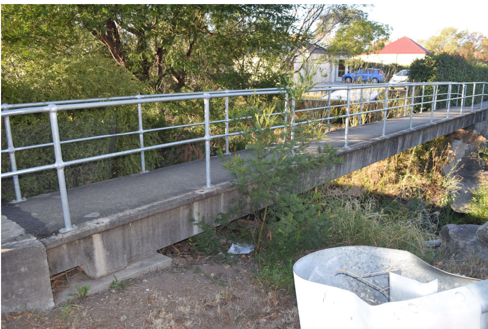
Figure 1 Perspective views of the road and pedestrian bridges spanning across Redbank Creek on Remembrance Driveway, Picton.
