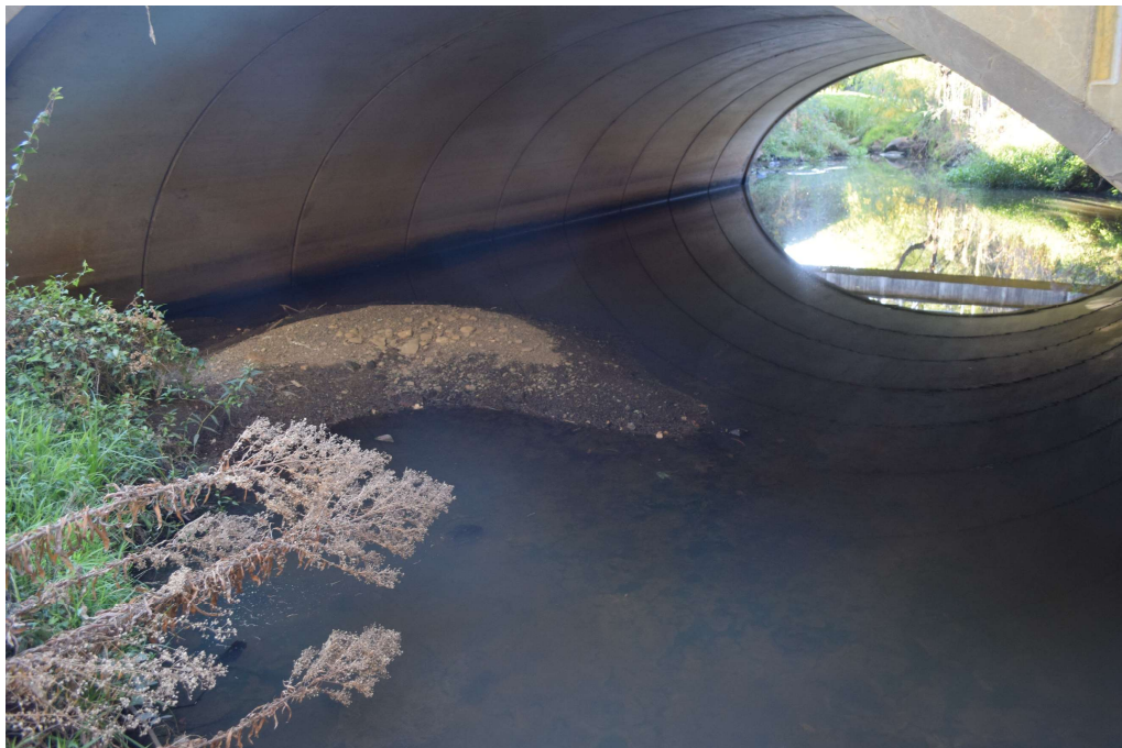
Figure 7 Ponded water below the road bridge during period of dry weather noting the sediment on the creek bed.
