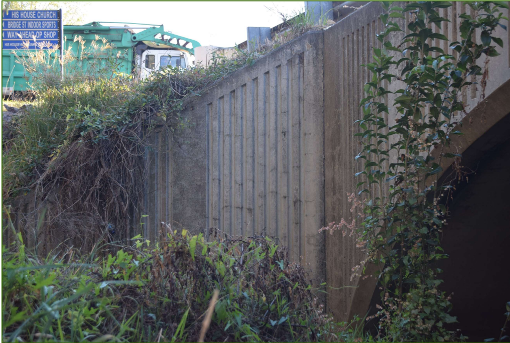
Figure 2 North-western precast concrete wingwall on Sydney abutment noting that the truck shown in the background is stationary on Bridge Street, where it intersects with Remembrance Driveway.
