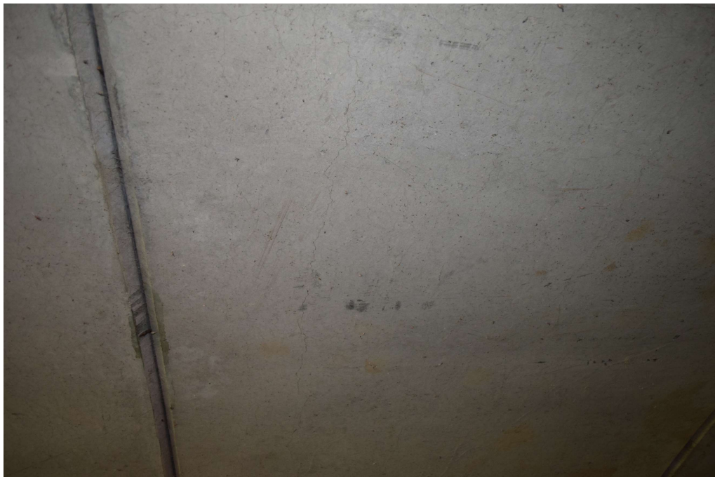
Figure 9 Hairline cracking observed on the intrados of one of the arch panels.
