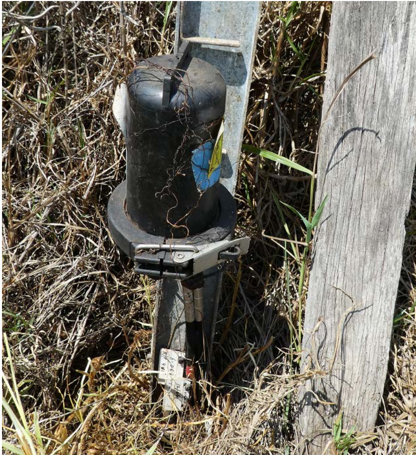
Plate 5: View of above ground joint 10Pr/6Pr in Stilton lane over LW31 showing direct buried copper cables entering above ground openable joint.
