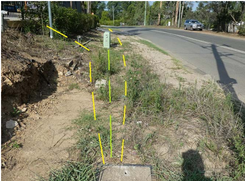
Plate 6; View east along Bridge Street showing Telstra optical fibre cable (yellow) to Energy Australia Depot in Bridge Street. Also shows cable feed into Redbank Place and NBN cable (green) to their Node from the Telstra Pit.
