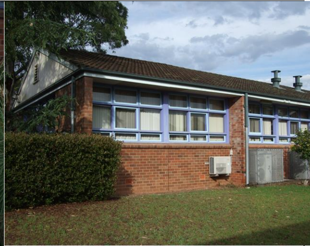
Figure 16 Block A gable wall has windows. Note vertical control joint in brickwork below window sill
