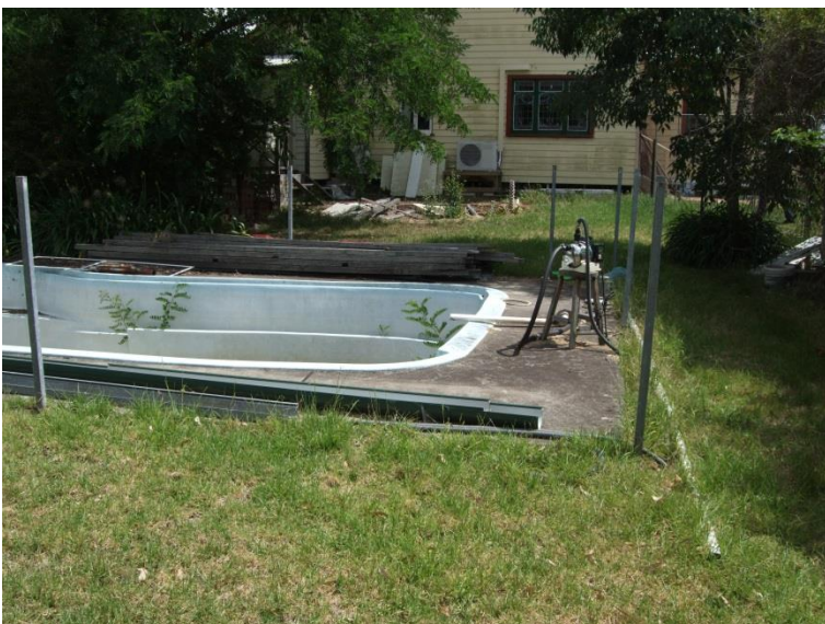
Figure 58 Dilapidated fibreglass in-ground pool
