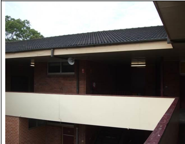
Figure 37 Block I PAR_210_pa09 & 08 at first floor showing slab movement joint reflected in balustrade
