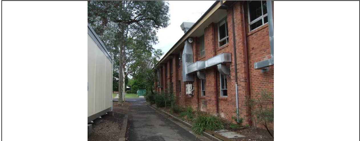
Figure 36 Block I PAR_210_pa10, two-storey load-bearing cavity brickwork structure, with suspended first floor concrete slab and a cruciform arrangement of movement joints, supported by a concrete ground and footings
