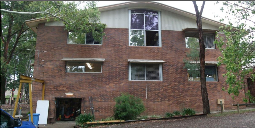
Figure 31 Block J PAR_210_pa12, two storey reinforced concrete beam/slab and column frame with perimeter articulated cavity brick
