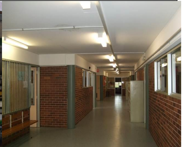
Figure 33 Block J PAR_210_pa12 ground floor showing beam/slab and columns and infill internal brick walls
