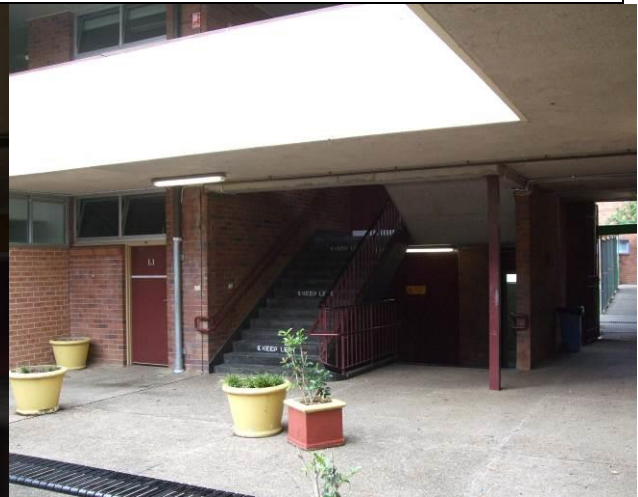
Figure 38 Block I PAR_210_pa09 & 08 at first floor stair up to first floor at western end of courtyard
