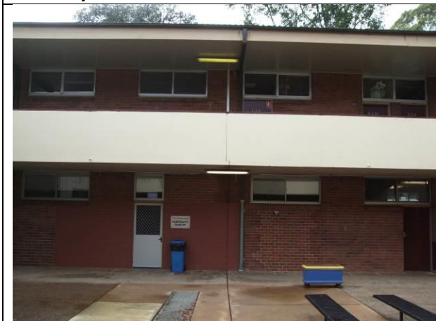
Figure 39 Block I PAR_210_pa10 & 09 showing movement joint, which is reflected in the ground floor brickwork and the ground floor slab
