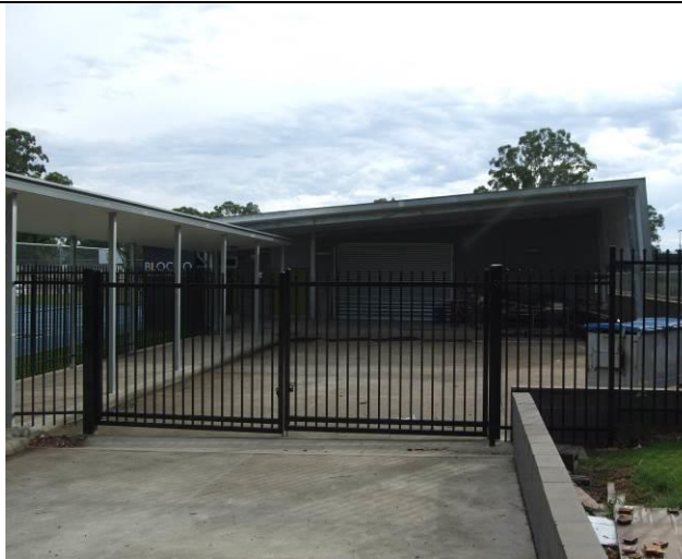
Figure 27 COLA structure PAR_210_pa15 with covered way roof structure PAR_210_pa38 in the foreground.
